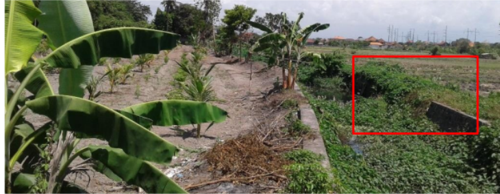
Figure 4. Damage in River Revetment and River Silting
